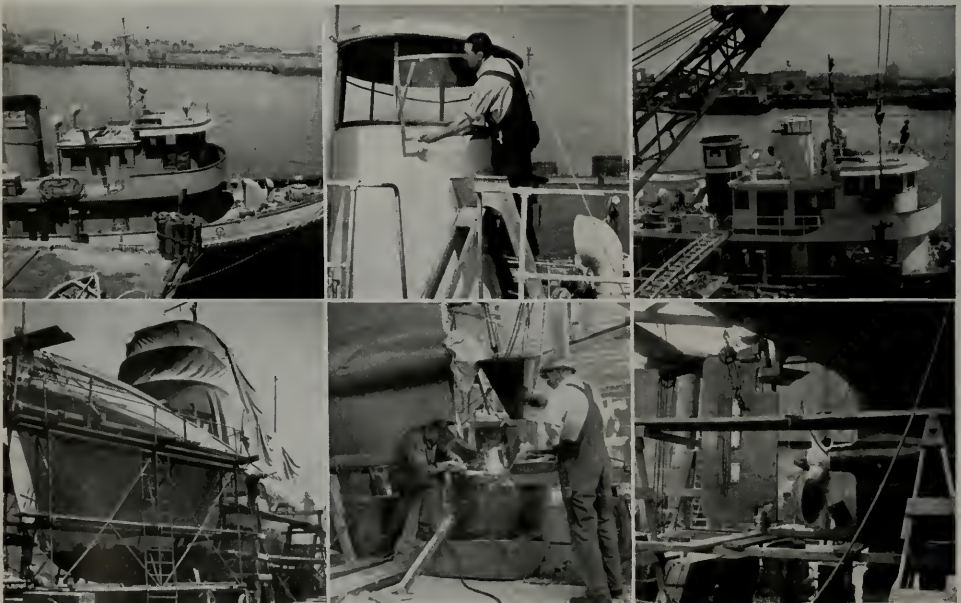
Atop, left: The Robert Gray as she looked before installation of her new observation tower. Center: Workman installing plexiglass window in observation tower. Right: The Robert Gray in her new coat of paint with her new observation tower virtually complete. At bottom, left: Sandblasting the hull on the Robert Gray . Center: Thermit welding new section of skeg for rudder, which was enlarged to give better steering control. Right: Stern section showing new skeg extension and enlarged rudder in place.
